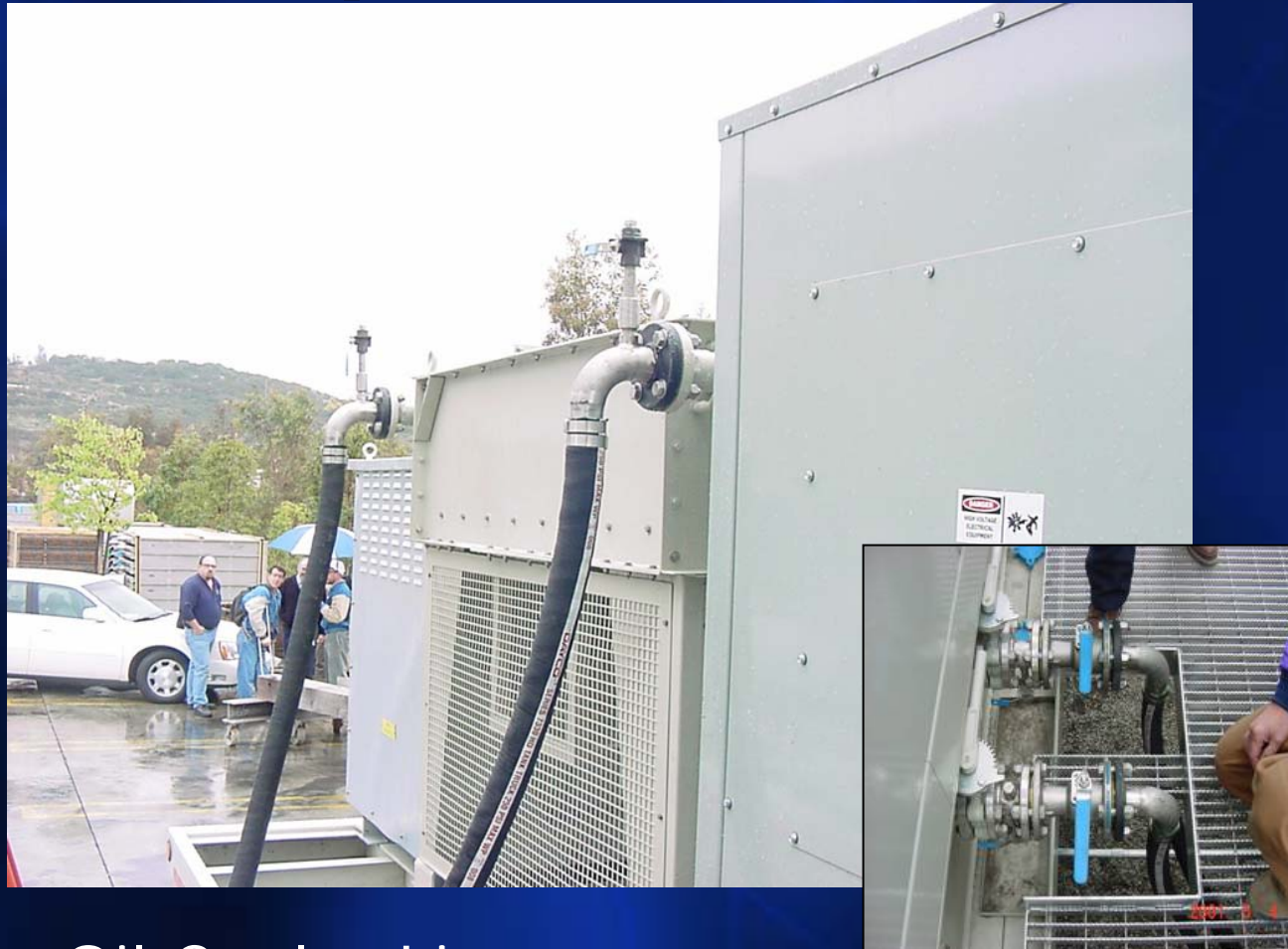
Oil Cooler Lines
