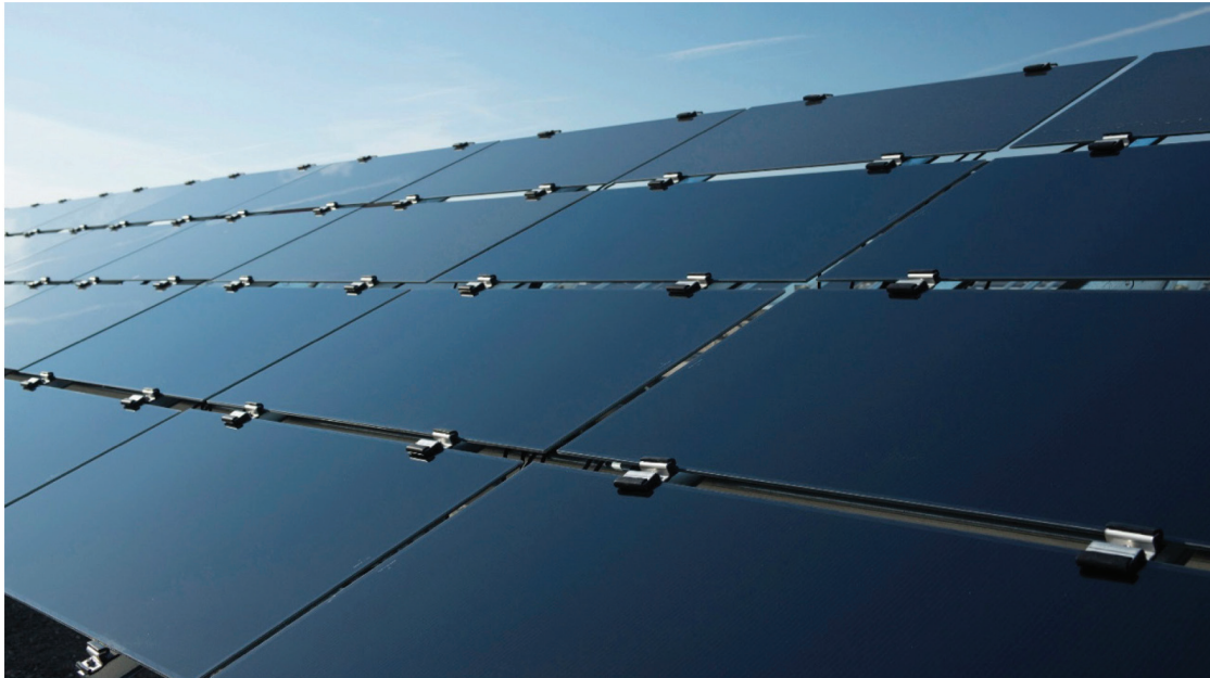
Figure 6. Typical thin-film PV array on racking system and clips
