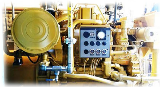
The new cogen engine, the heart of the Cogen Expansion Project
