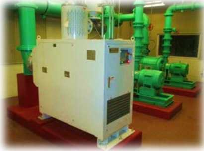
New high speed turbo blower (foreground)
