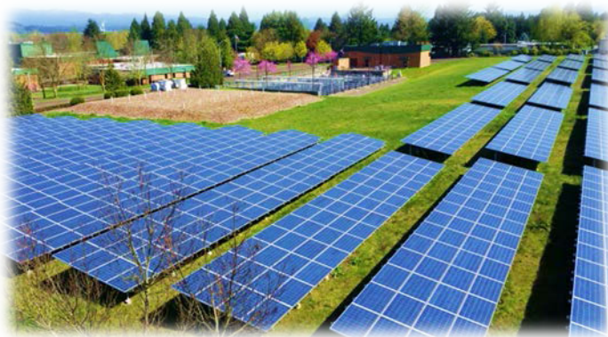
420 kW solar array installed in 2009, at the time of installation, the largest in the NW
