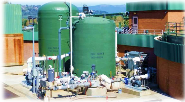
Expanded FOG Receiving Station
