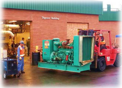
Removing old standby genset. Notice cut out (right) for new garage door in Digester Control Building to accommodate second cogen unit
