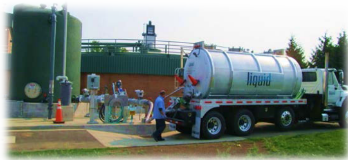
FOG hauling truck unloading at FOG Receiving Station. (Anaerobic digester in background)
