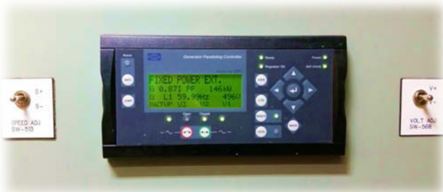
Deif paralleling controller matches cogen output with grid power
