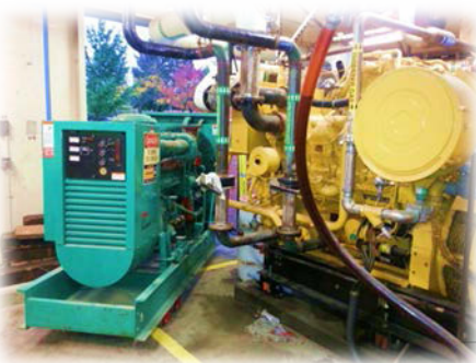
Removing old standby genset from digester control building to make room for new, second cogen unit
