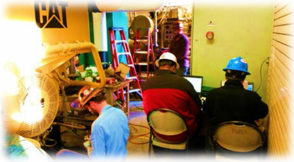
CAT technicians using laptops to program and test system during startup, January 2015
